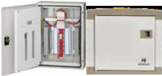
Distribution board and panel box
